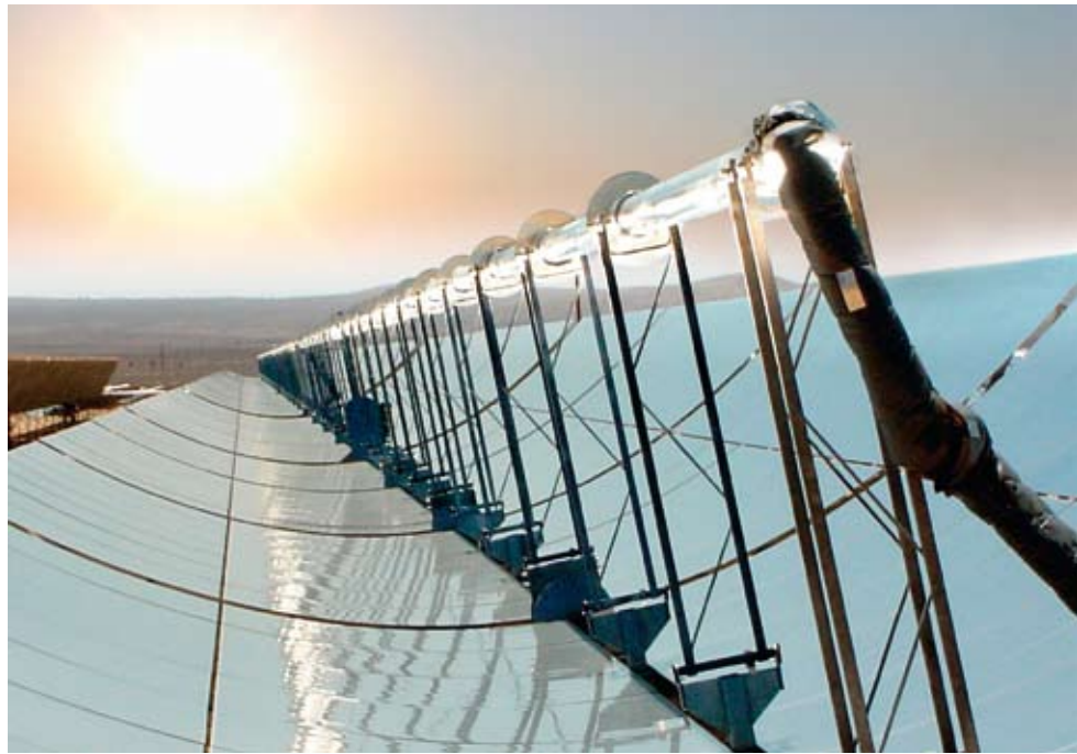
Close up view of parabolic trough and heat collector.
